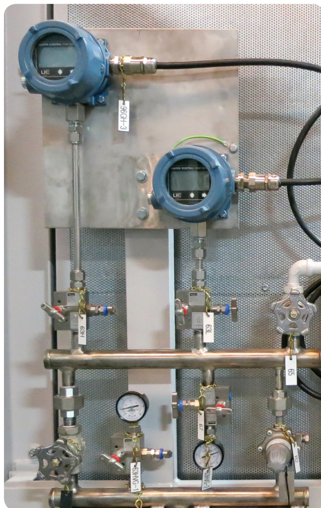
Seal Pressure Monitoring
