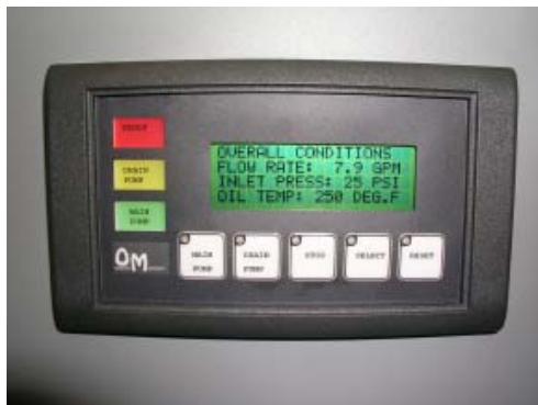
The local operator interface panel displays the system's operating status at all times.
